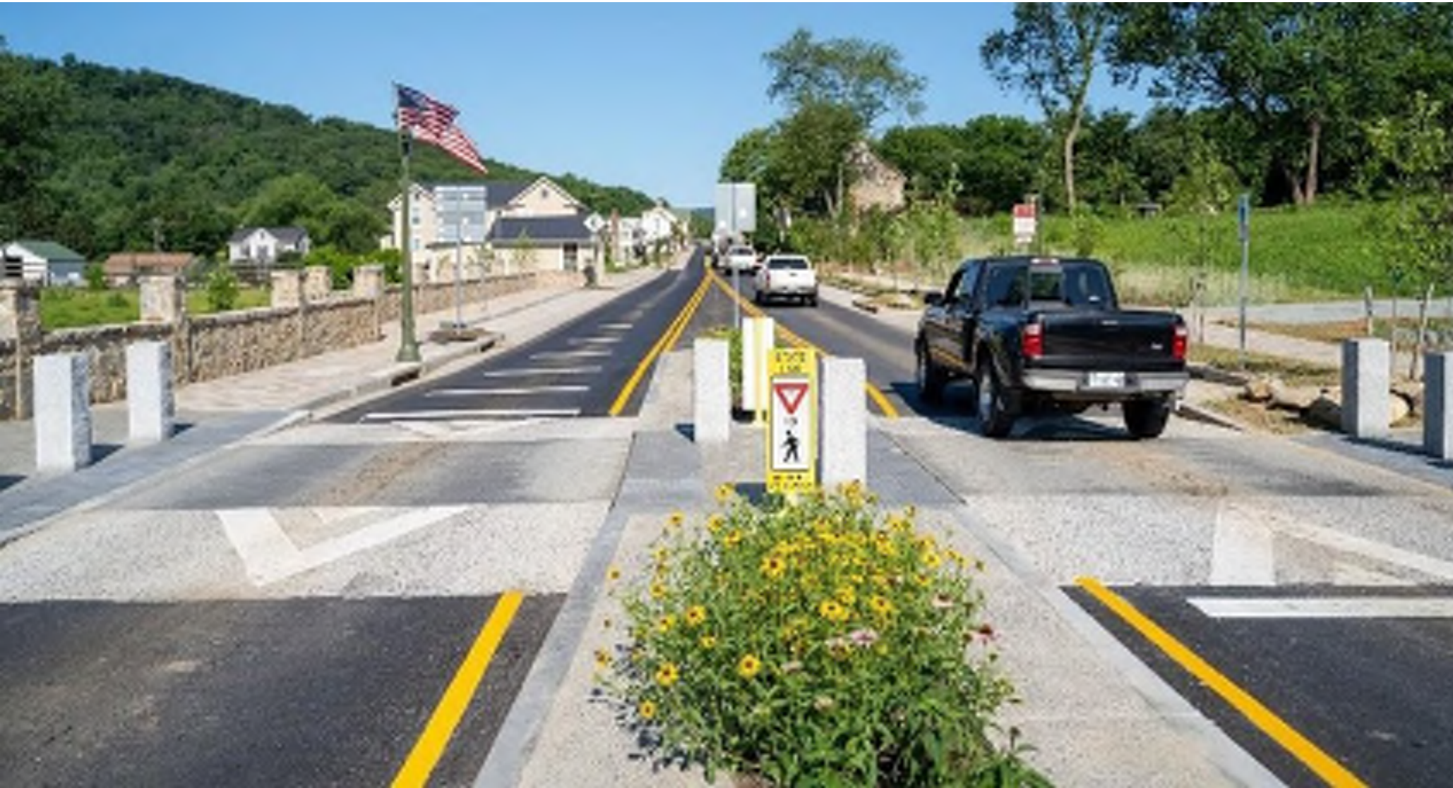
Pedestrian accommodations are incorporated for people to cross the road safely and reach destinations by foot comfortably.
