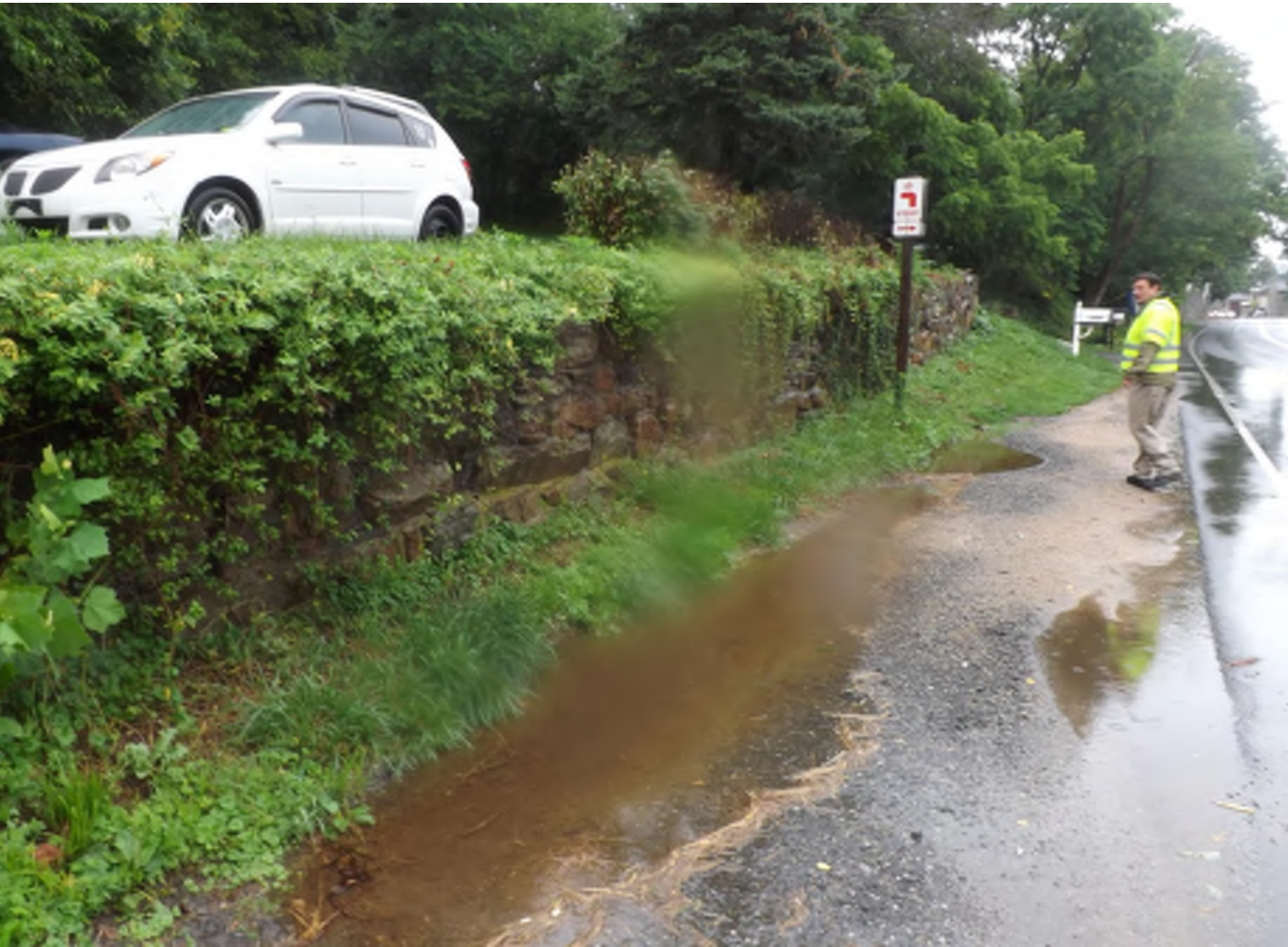
Inadequate infrastructure and challenging topography
