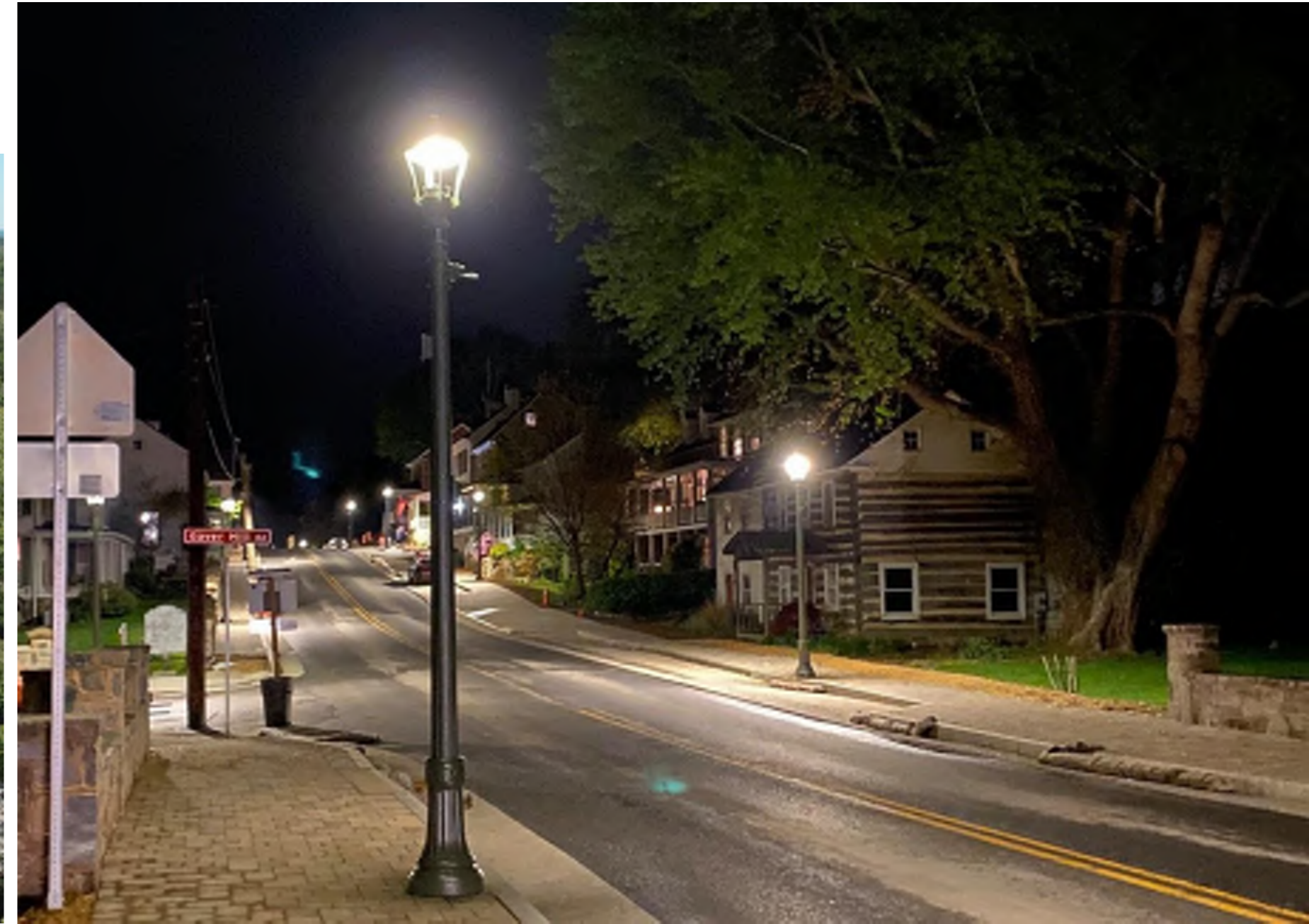
New lighting provides safety at night. Full cut off LED lights with side shields.
